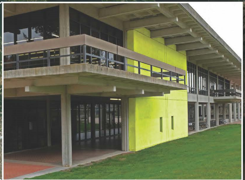
This is just one of the many seismic mitigation projects completed across the Evergreen State College campus. In this photo you can see the shear wall (highlighted in yellow) that was installed to reduce lateral movement of the building during seismic events.
