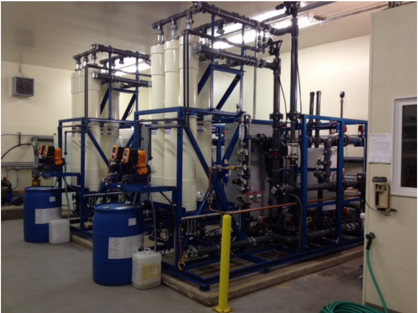
Water Plant Membrane Skids
