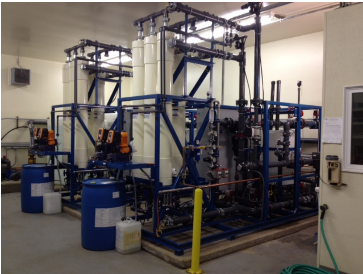
Water Plant Membrane Skids
