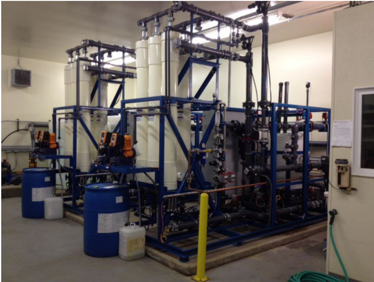
Water Plant Membrane Skids
