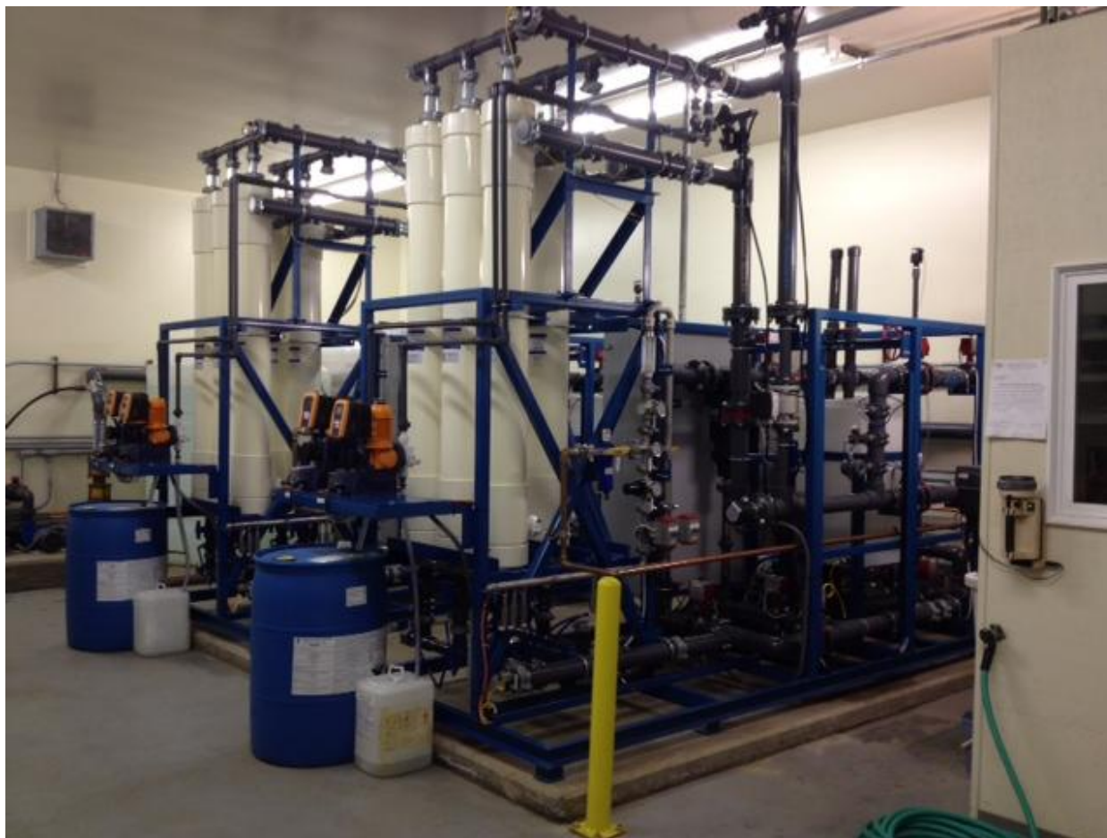
Water Plant Membrane Skids
